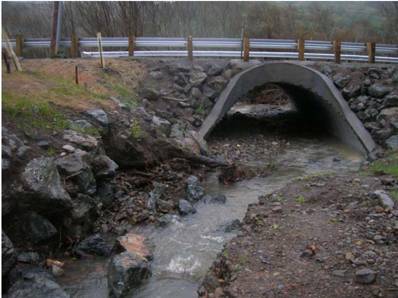
Figure 3. Restoration of the natural channel allows the passage of salmon as well as woody debris, which could block this undersized culvert and cause flooding of the roadway.
