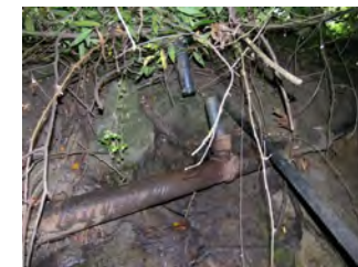
Investigating a resident's complaint about soapy water in a creek, County stormwater staff discovered this broken sewage lateral. It was repaired the next day.
