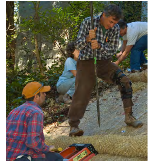
Installing an erosion control blanket at MCSTOPPP's creek bank restoration workshop (see page 6-1). Photo by Sam Wilson
