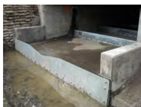
Baffles were installed in this box culvert, and the downstream channel of Vineyard Creek was stabilized, to aid steelhead in passing upstream during high flow conditions. Project completed October 2008.
