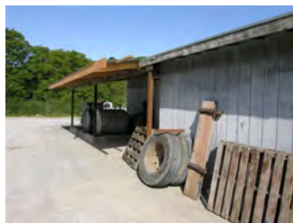
An industrial facility owner added this shed roof over stored hazardous liquids following an inspection.
