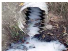
Paint and concrete slurry are among the most common illegal discharges.
