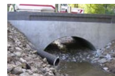
Arched culvert being installed to facilitate fish passage on Woodacre Creek at Park Street in Woodacre.
